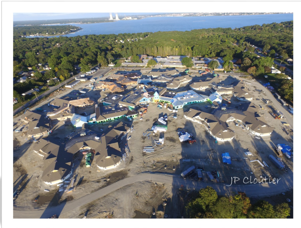
An aerial photo of the RI Veterans Home project taken in October, courtesy of JP Cloutier and his drone.
